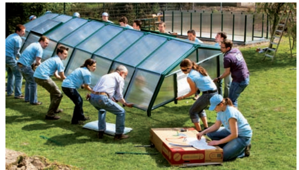
Trainees from the International Graduate Programme building a greenhouse for a school
